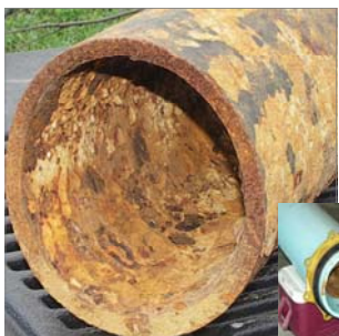
8" Pipe Before RE-Ox Treatment
