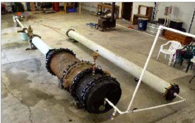
The first Pilot Trial consisted of pipe and valves taken from service and assembled to receive the flow of RE-Ox treated water.
